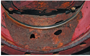
Improper continuous use of butterfly valves as a control valve can result in dramatic material damage, as in this valve opened by 5° after a year in seawater.
